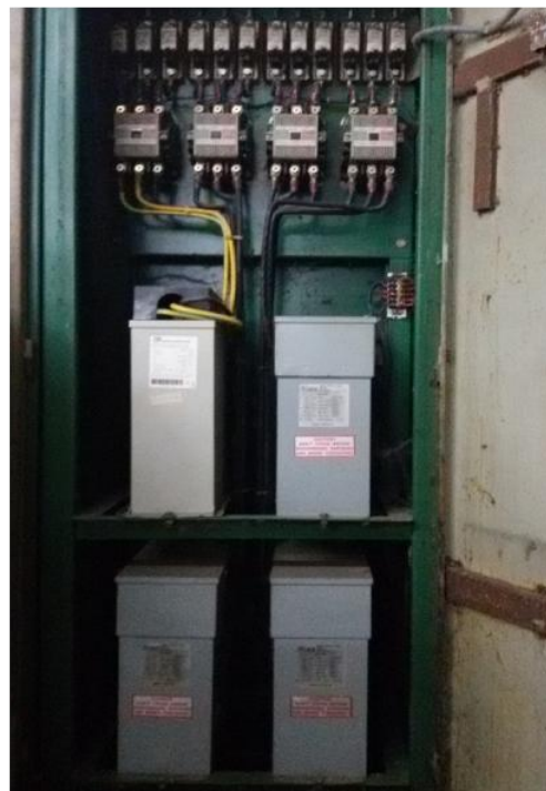
Panel CB Winding Patal II
