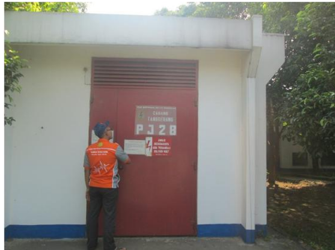
Gardu Distribusi pabrik (PJ28)
