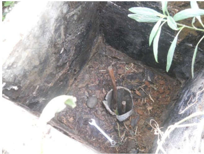
Gambar 4.20. Bak Penacapan Grounding SS-3
