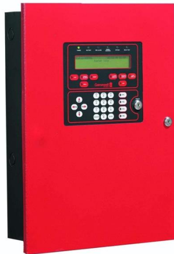
Gambar 2.6 Fire Control Panel
