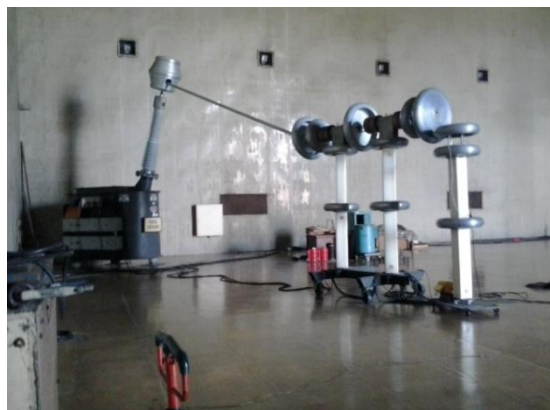
Gambar 3.15 partial discharge test set
