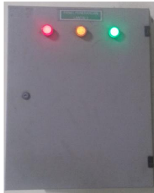
Gambar 2.6 Panel (Sistem Kendali Manual Instalasi Penerangan)
