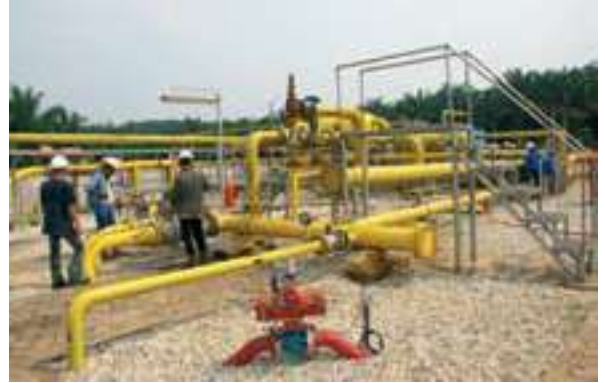
Gas Production Facilities (Korinci Baru PSC)
