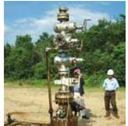
Gas Well Head (Suci OCA)
