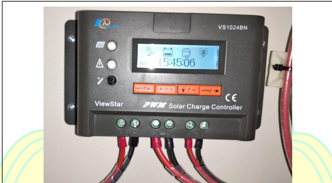
Solar Charge Controller
