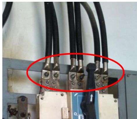
Gambar 2.1. Unit Masukan ( Incoming ) PHB TR
