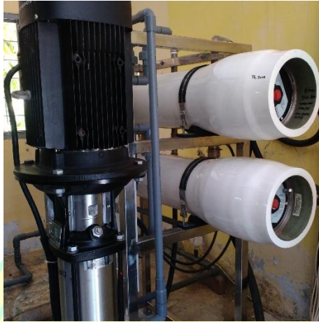
Filter air RO ( Reverse Osmosis ) di Pulau Untung Jawa
