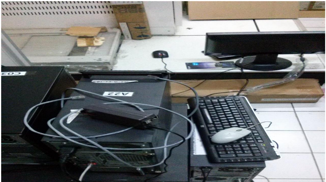
Server Streaming Video gedung D Ruang Server Pustikom
