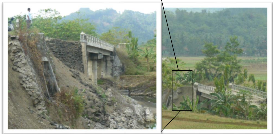
Gambar 4. Tebing jembatan longsor
